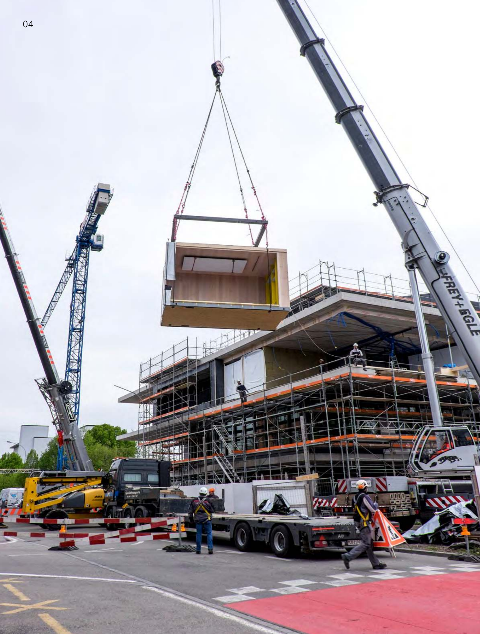
Installation of the prefabricated modules for the unit Vision Wood on April 26, 2016.
